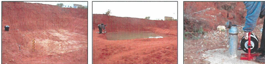
Figure 3 – Infiltration basin in the second layer and monitoring equipment used for the infiltration test
