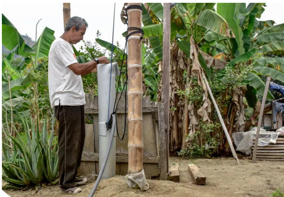
Figure 8-7: The well installed at home. Water and Sanitation Program in dispersed rural communities in the Canton of Portoviejo, Province of Manabí, Ecuador.
